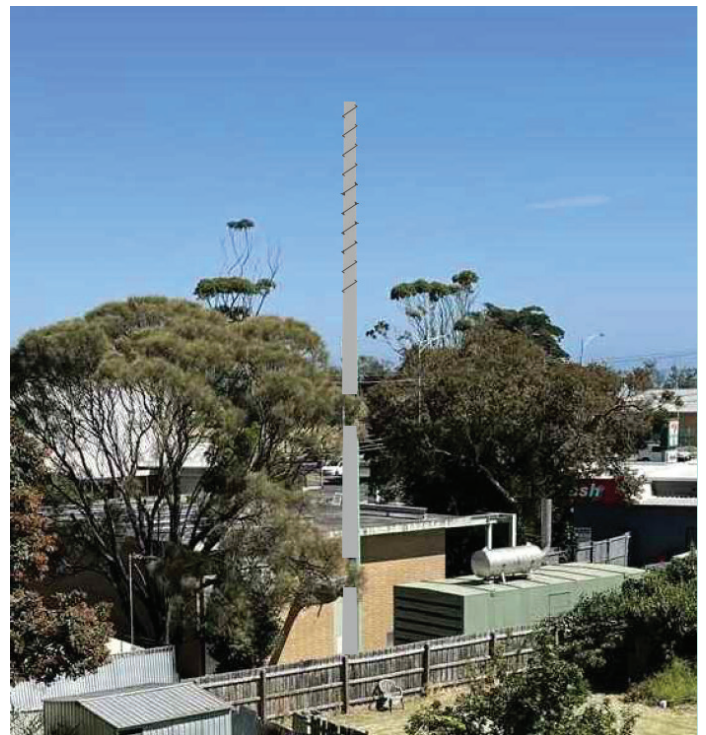
New 15m tall stack viewed from south-east of the pump station.
