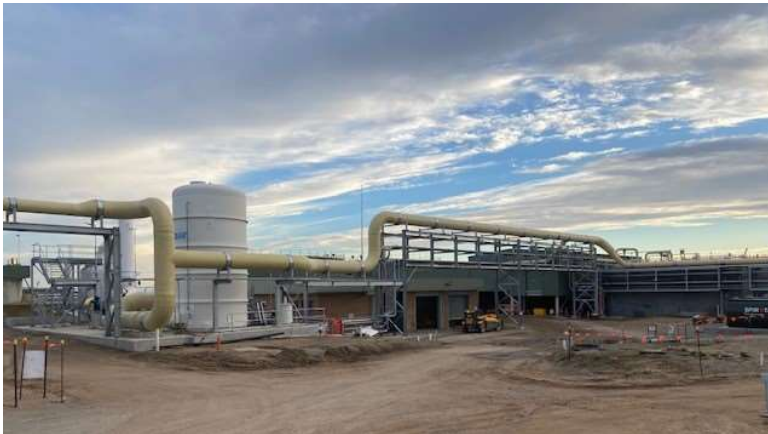
Above: Odour ducting and management system.
