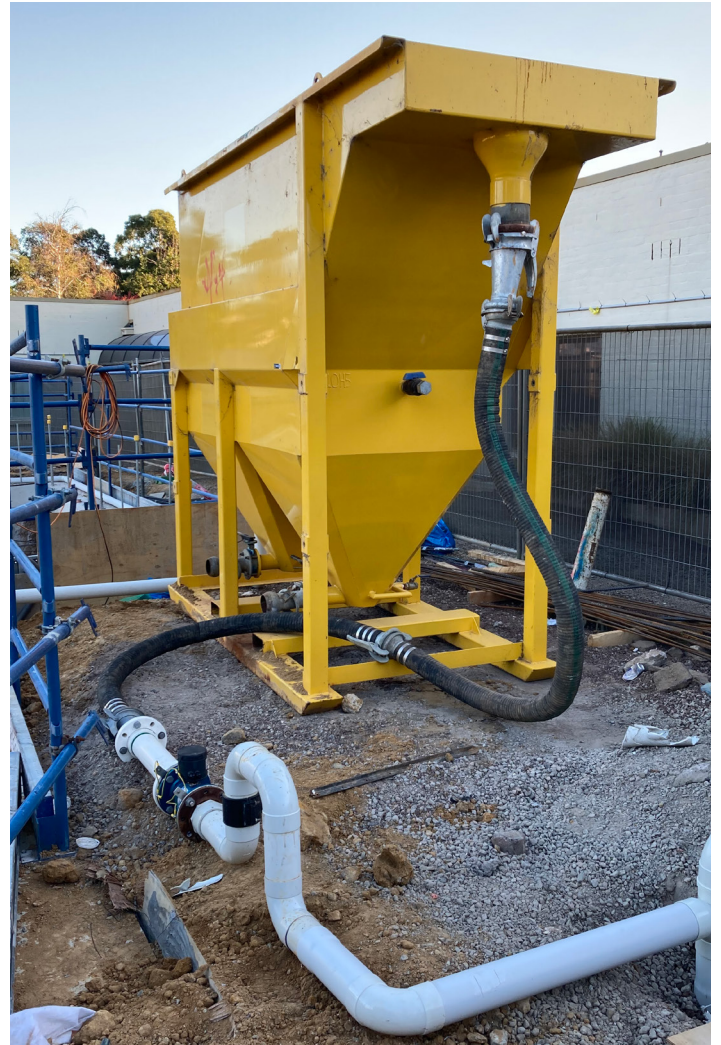
Settling tank and electromagnetic flow meter
