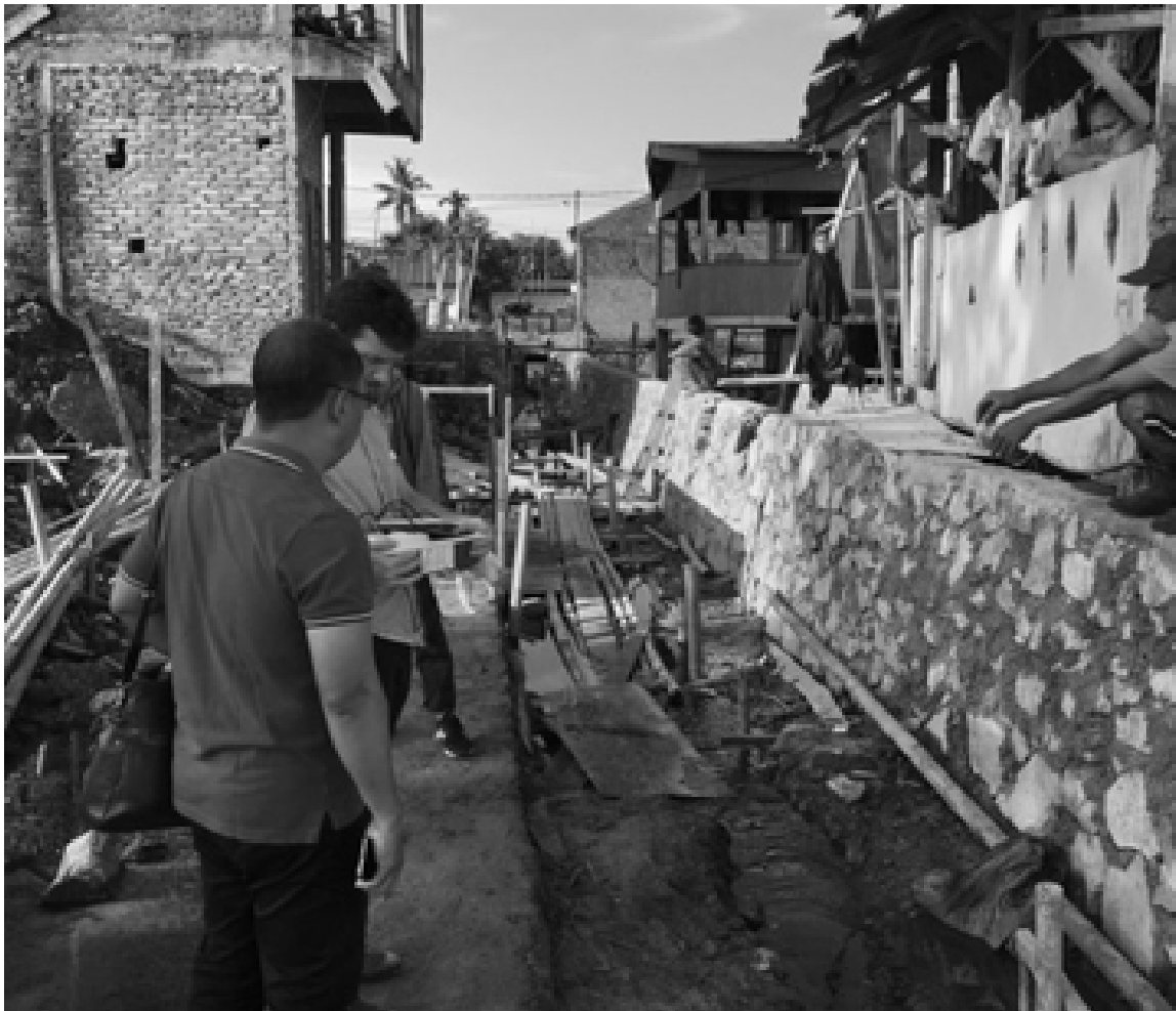
Iota's Technical Director, Eamon Casey in Suva, Fiji. He's demonstrating how to use Iota's OneBox® devices to control wastewater flows.
